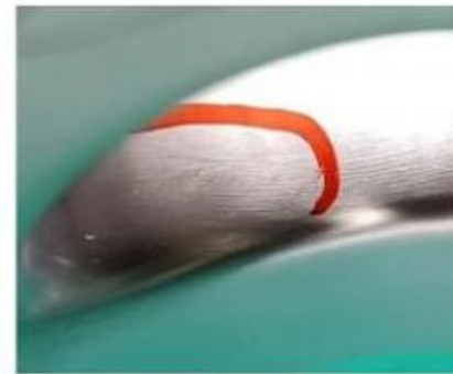
09. The weld bead is not clean, unqualified
